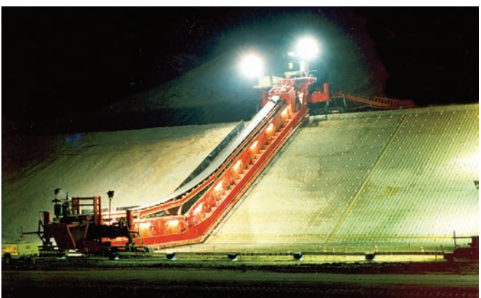
▲ Night lighting system illuminates not only the G&Z Canal Liner but much of the surrounding area.
