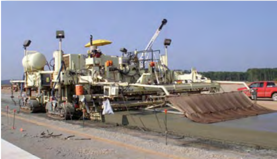
Lane paving at Dulles International Airport in Dulles, Virginia with G&Z's S850 and Compact Dowel Bar Inserter. Paving width at 18'-9" (5.71m), 17" - 17 1/2" (432mm - 444mm) thick concrete pavement. 1 1/2" (38mm) diameter dowels, 20" (508mm) long dowel bars on 18" (457mm) centers.
